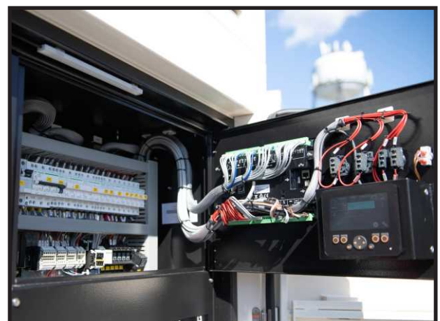
Easy access to labeled wiring and breakers
