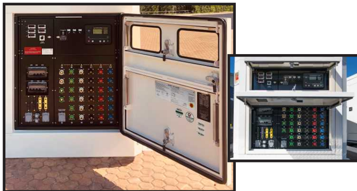
Control panel with two door opening options
