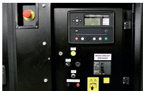
Control panel, with Deep Sea Controller, laid out and labeled for easy use. (other brands available)
