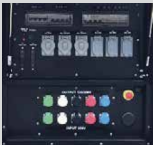
Protected outlet panel
